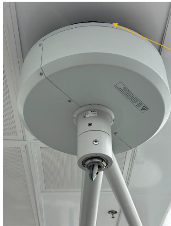
Image 3: Example of a ceiling cover that is not flush with the ceiling
