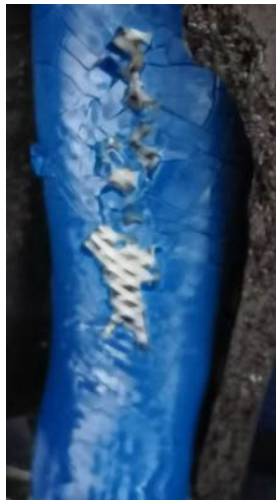
Figure 1: Degraded drain hose
