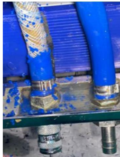
Figure 2: Degraded vs. intact blue colored hose
