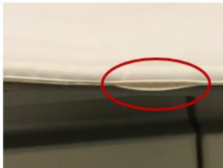
Figure 1 example of separated seam
